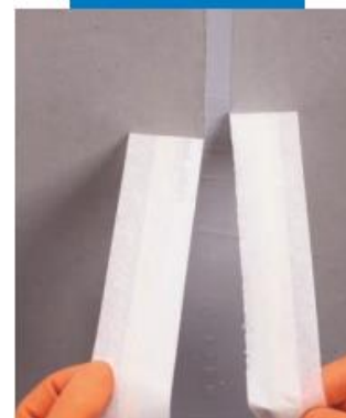
Removal of the masking tape applied around the edges of the joint to avoid rough edges
